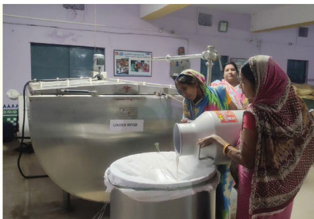
Two thousand litre Bulk Milk Cooler at Roth, Block - Agalpur, Bolangir, Odisha under NPDD
